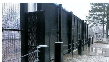
USA Tier 1 Substation
